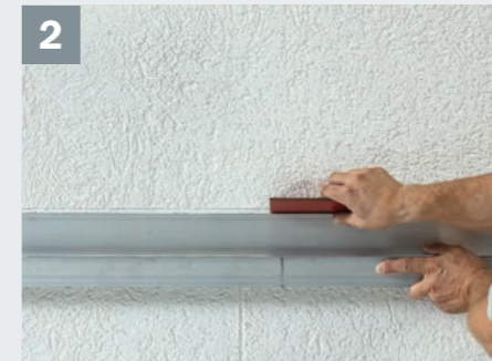
2 ...and the joint pattern according to the joint plan in created with the desired joint width. We recommend using an H Rule (thickness 6 mm). The maximum field size of the individual sections is 10 m 2 .
