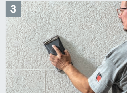
3 After standing for 24 hours* roughly sand the surfaces and joints with 16-grit sandpaper.
