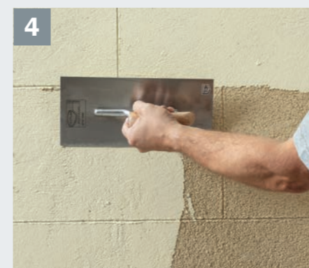
4 Then the grain structure is covered with Baumit CreativTop Pearl in colour shade 0217 almost completely filled without taking into account the pre-jointed joints and rubbed down smoothed again with light pressure or rubbed in with a steel trowel. Defects or air voids contribute to the imitation of a sandstone surface.
