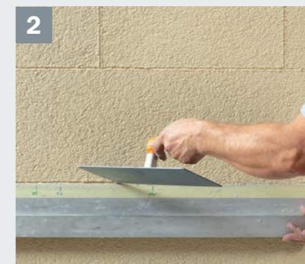
2 ...and the joint pattern created according to the joint plan in the desired joint width. The use of an H Rule with the help of a plastic float is recommended here.
