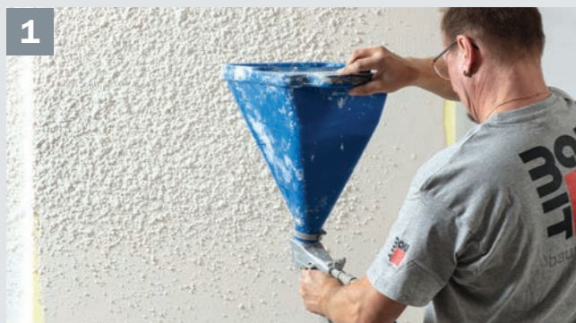
1 Baumit CreativTop Max is applied crosswise evenly to the substrate. A field delimitation is to be implemented if, due to the local conditions, no uninterrupted structuring of the entire area can take place.
