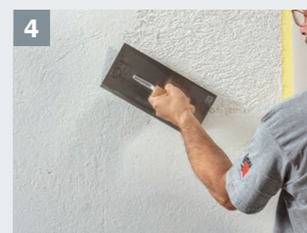
4 Subsequently, the grain structure with Baumit CreativTop Pearl is filled all over the surface and smoothed again with light pressure without taking into account the pre-joints. rubbed with a steel trowel. Small flaws or air voids help imitate a concrete surface. After stiffening, the joints are restructured again using a plastic float.
